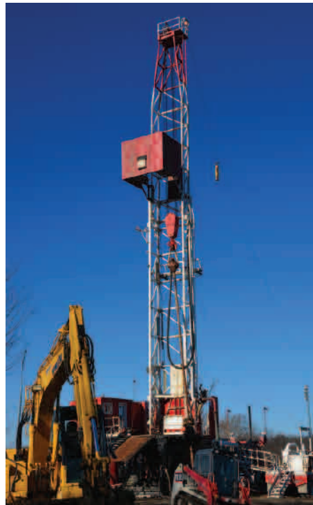
The drill rig tower stands 120 feet in the air. (right) The drill rig in Holiday Park.
