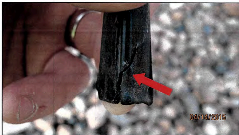
Figure 3: The vinyl weather seal was very brittle and split during the removal of the seam cap (area shown with red arrow).
