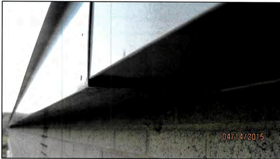
Figure 16: North Elevation, it appears ice buildup has damaged this joint.
