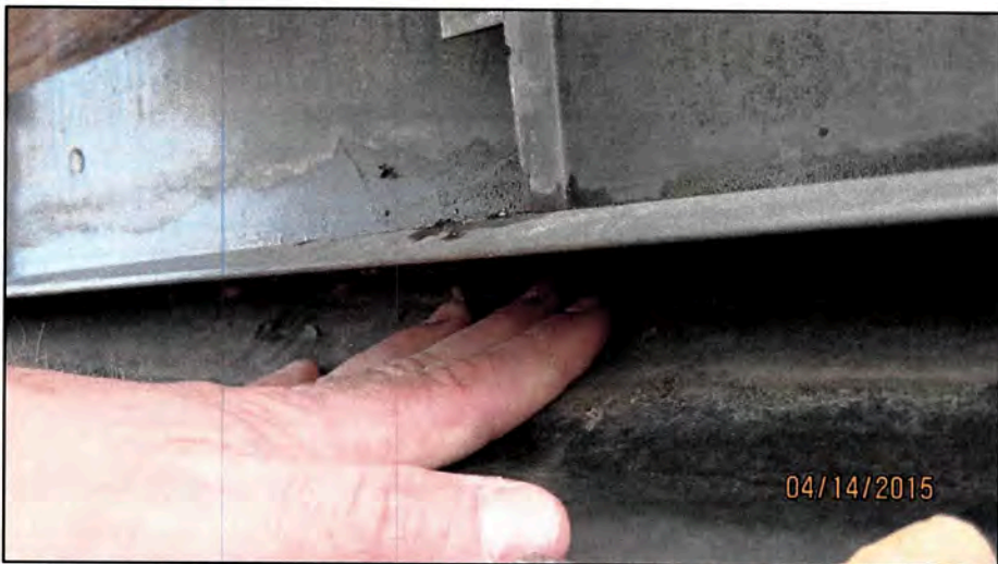
Figure 5: The Mansard panels sit on the sill flashing shown above my hand; the EPDM membrane terminates behind the treaded lumber.
