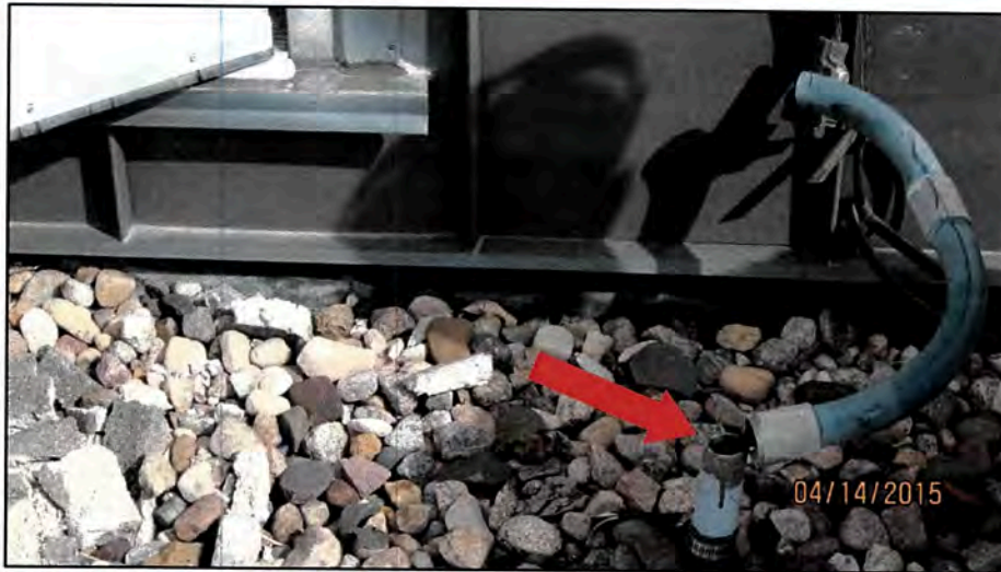
Figure 12: The lightning protection system conduit is not permanently sealed (area shown with red arrow).
