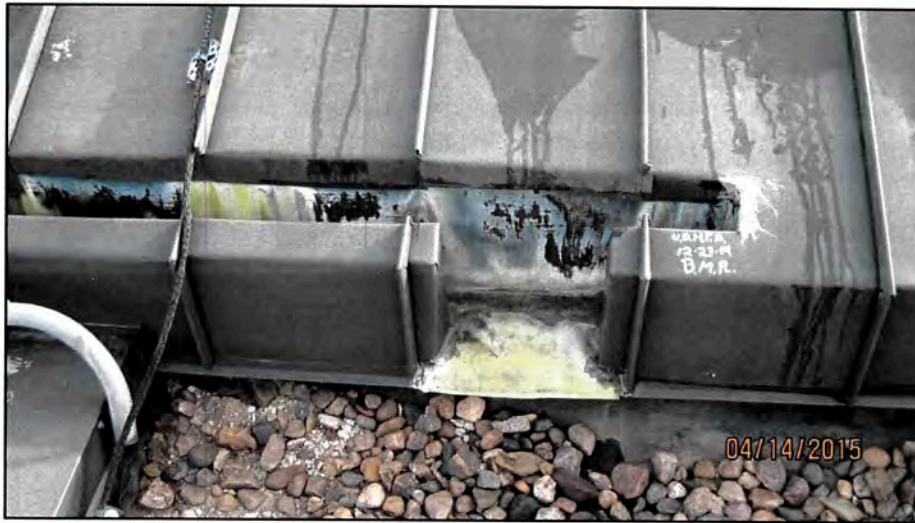
Figure 6: The internal gutter system that is located at the main entrance of the LEC.
