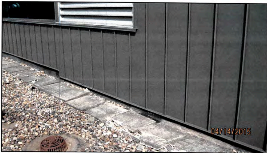
Figure 4: East Elevation, these vertical Tee-Panels will need to be field cut to allow for the installation of the new roofing system.
