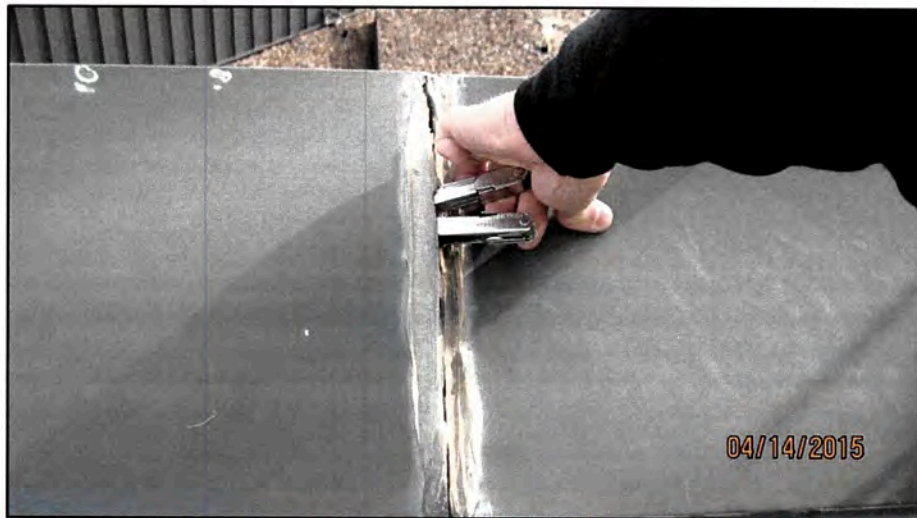
Figure 9: Additional image of the two-piece ridge cap flashing. The majority of the field joints are not permanently sealed.
