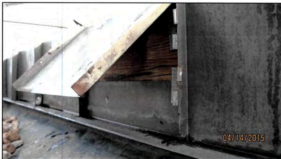
Figure 2: One Mansard panel was removed to review the sill flashing installation and the EPDM membrane termination.
