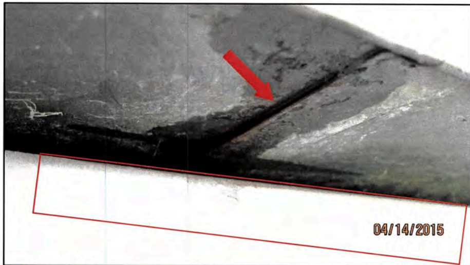
Figure 17: North Elevation, the Mansard sill flashing joints (area shown with red arrow) are allowing moisture to migrate behind the box gutter (area outlined in red).
