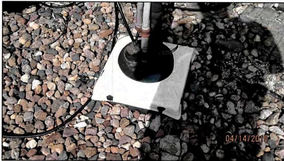
Figure 14: Some of the mechanical curb heights need to be raised.
