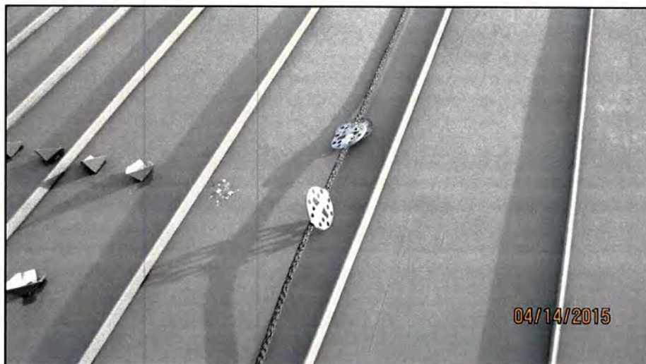
Figure 11: The adhesive base plates are not adhered to the Tee-Panels.
