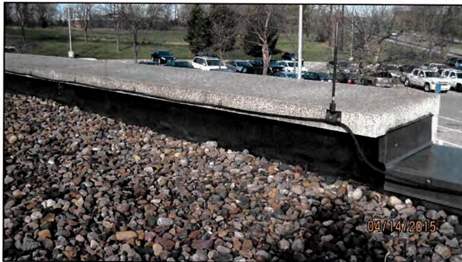
Figure 7: Sally Port Roof, the concrete coping caps are starting to deteriorate.
