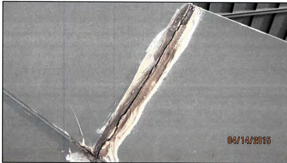
Figure 8: Two-piece ridge cap flashing, the exterior control joint sealant is completely separated.
