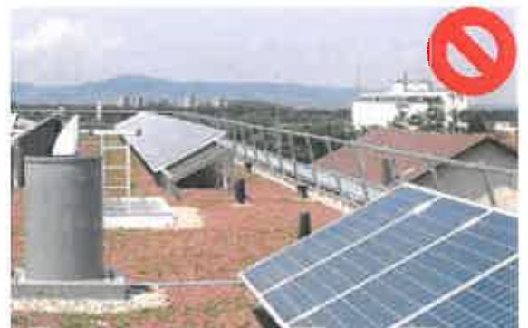
Incorrect: Panels are installed close to roof edge requiring a fall protection railing
