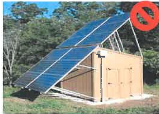
Incorrect: Framework is not fully enclosed
