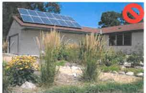
Incorrect: Panels are mounted higher than 1 foot from roof surface
