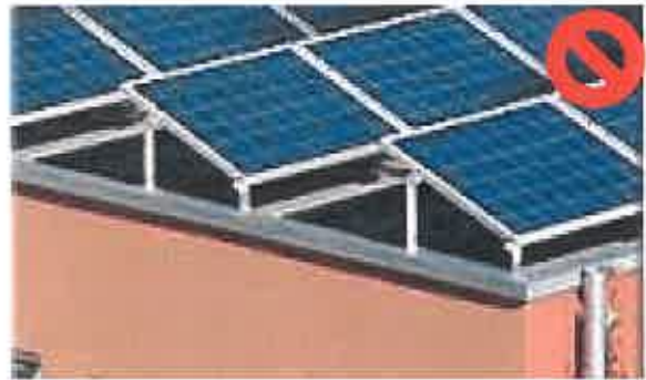
Incorrect: Panels are too close to roof edge
