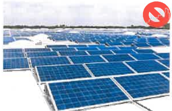
Incorrect: Not consistent, gaps in arrangement
