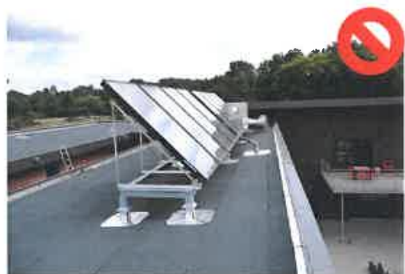
Incorrect: System height greater than 7' above roof
