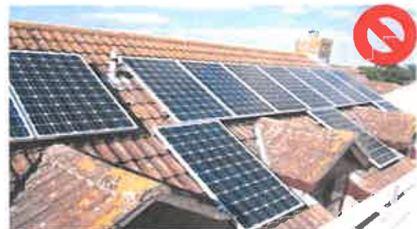
Incorrect: Not consistent, gaps in arrangement
