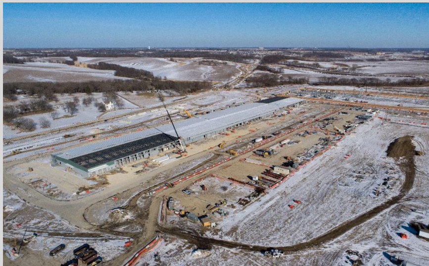
Microsoft Data Center Site – 11100 Boonville Rd.
